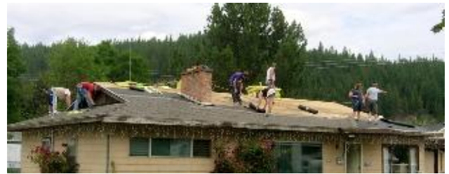
Shoshone Base Camp Servants join with Fuller Center workers in a "Greater Blessings" project to roof Karen North's home in Pinehurst. On the far left is SVFCH President, Mike Humphrey & on the far right is SVFCH Supervisor, Kevin Hutchings.
