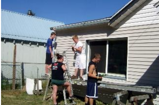
Pilgrim Lutheran Church youth from Puyallup, WA, work on the front of Darnell's home. Photo by Judy
