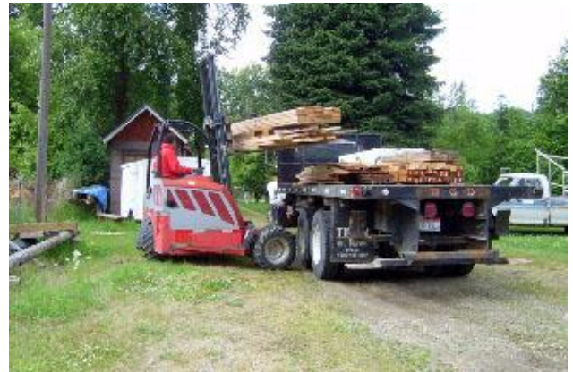
Dale Jacobs delivers a large lumber donation from Kellogg Lumber Co. Photos by Judy
