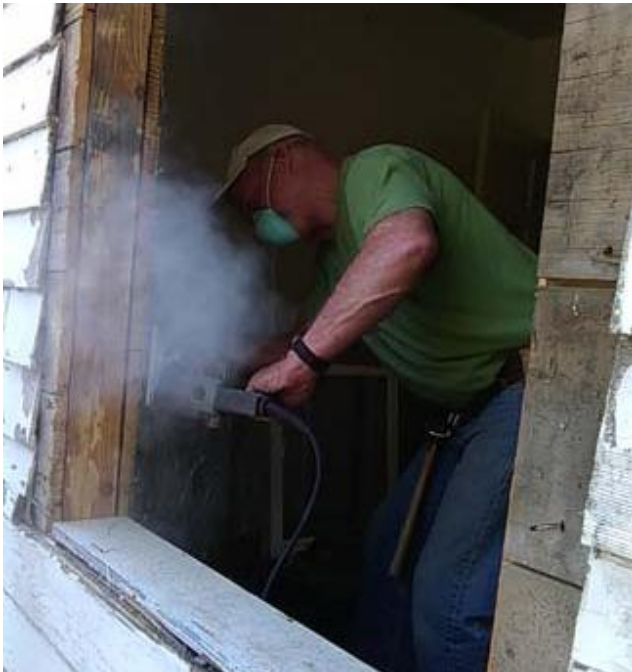
Rick Gilbert prepares the opening for a new window in the Osburn home. In the process, he uncovered part of the interior wall to discover that there is no insulation between those walls.
