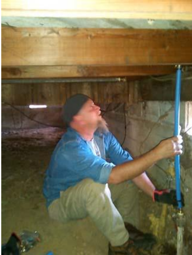
Randall Rosson works on plumbing under the Osburn house. A hot water tank needs to be installed before water can be turned on to check for leaks.
