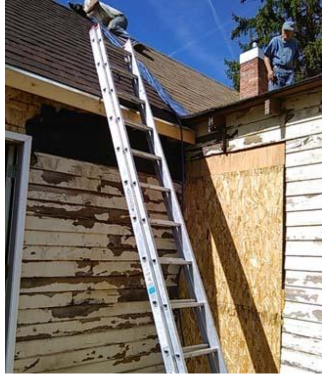
Sam Wiget, a volunteer roofer, installs the shingles to cover the tar paper used by the Michigan Servant Adventurers last month. Verne is safety supervisor and serves as gofer.
