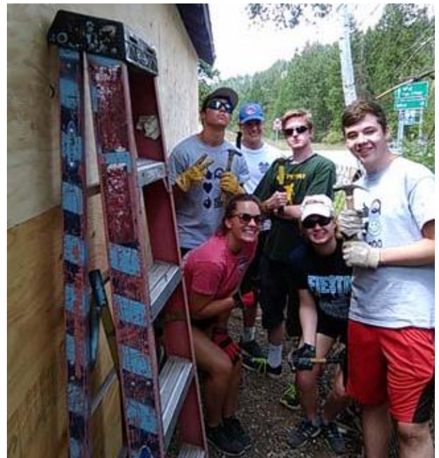
Another crew of Servant Adventurers installs new siding to replace the rotten boards on the garage making it a secure storage building.
