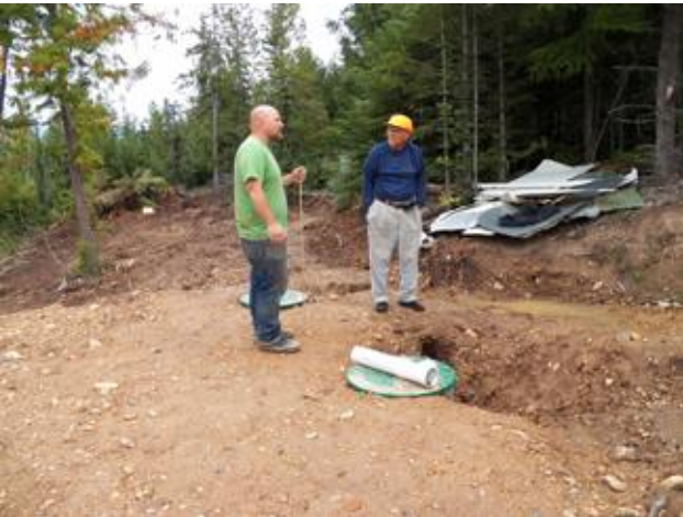
Joshua Mace shows Verne where the new septic tank is installed and where the drain field will go. The Mace site has been rewired; pump installed; and help lined up for building the framework to set the trusses on. We will be helping them with the trusses as a Greater Blessings Project.
