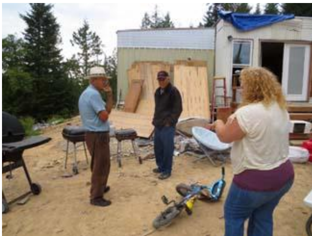
Verne & Carl Blalack discuss with Christina Mace how the trusses could be lifted onto the Mace home. The area along the sides is not wide enough for Carl to use his boom truck.
