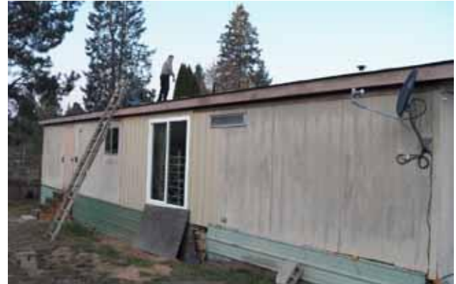
While Rick Wood kneels to hold the end of the tape, Steve Bourgard, of Bogie & Sons, measures the roof on Debra Bornitz's home.
