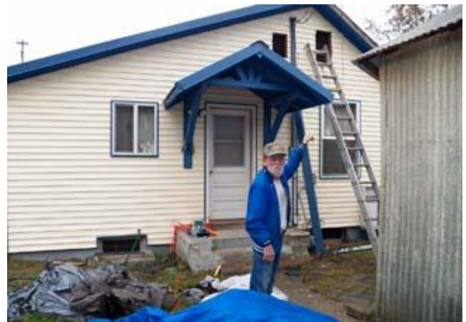
Work continues on Bob Larson's home where CJ Evans finished installing the roofing and soffits and is now ready to install insulation through the upper vents. Inside, Bob has been repairing the ceilings that had water damage when the tarp blew off in a violent storm.
