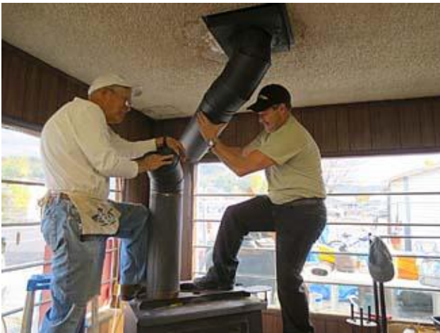
Verne asked Kevin Hutchings, when he was home, to help assemble the new stove pipe on the fireplace at the ReUse Store. Kevin is now working in Portland with Alaska Air. Glad to have the wood heat again. ☺
