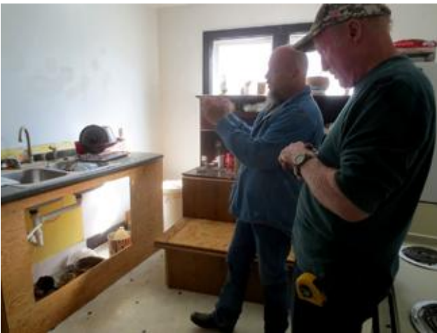
Randall Rosson and Rick Gilbert evaluate the need to replace plumbing under the kitchen sink.
