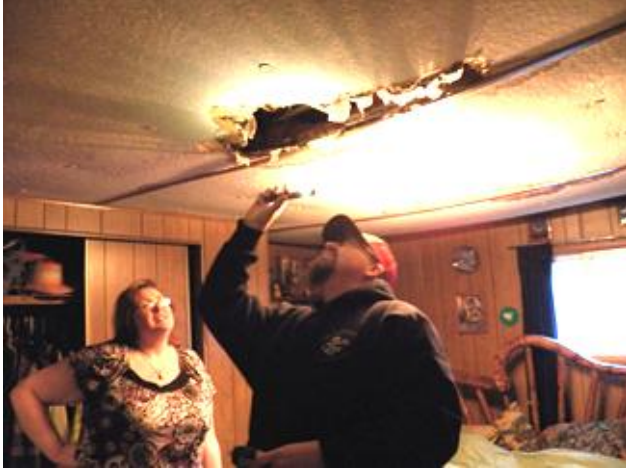
Krista Kirby watches as Kip McGillivray checks the wet insulation for mold.
