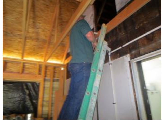
Rick Gilbert checks the location of the new furnace that Jeff Crawford of Systems Design installed in the Osburn house.
