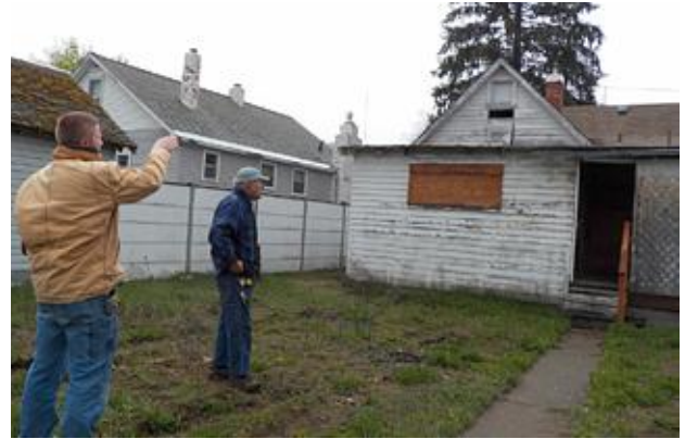
Clint Kunze and Verne survey the flat roof that is leaking in the laundry room. Verne is planning to get a building permit to extend the gable roof this direction so Clint's large crew with a supervisor can install it. Photo by Judy
