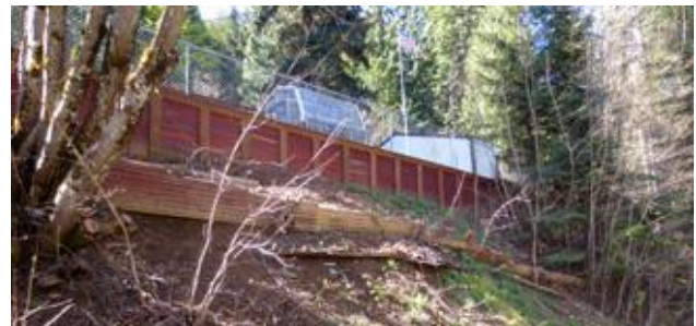
Our next GB project will be to repair a retaining wall for Donna Marquette in Wallace. Jim Taylor will ramrod the efforts with the help of the Holy Family Catholic 8 th grade graduating class from CDA. We need some volunteers to set a couple posts before they come June 5 th . Call Judy if you can set them. (Concrete must be mixed in a wheelbarrow.)
