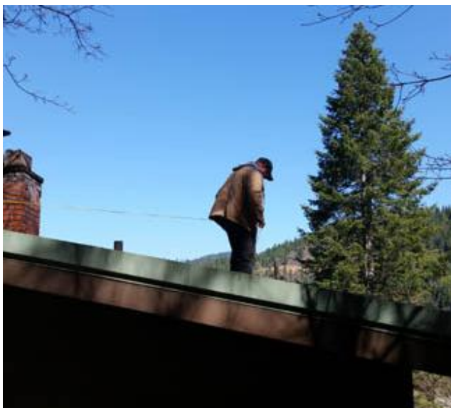
Jim also checks out Donna Marquette's leaking roof. He will fix the leaks on the main roof, but we need someone(s) to repair a damaged corner. Jim said he was too old to be doing that on a ladder anymore. We truly appreciate all the help Jim has given over the years.
