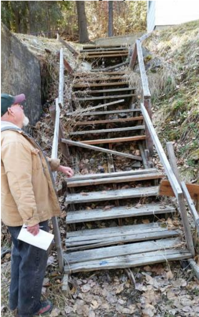
Jim Taylor checks out Nancy Elliott's steep stair on High Street in Wallace that needs replacing. We will provide materials but need construction volunteers.
