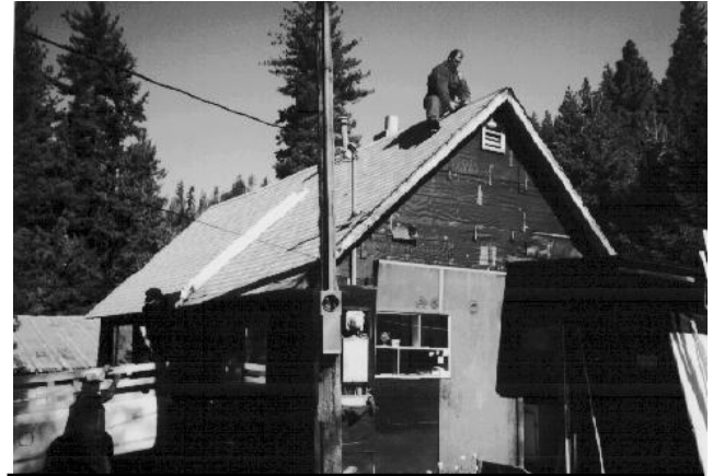
Bob Lane tears the first boards off the roof of his old house while George Shadle and Jim Shadle start up to help him. Photo by Roger Fulton
