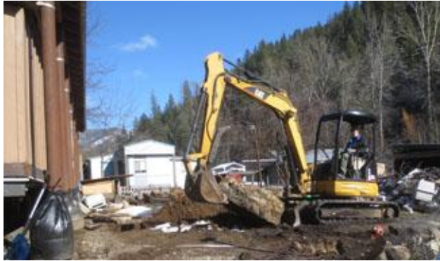
John Hopper brings his mini excavator to Krista Kirby's trailer site to fill in the hole. Photo by Judy
