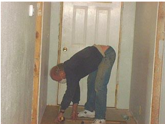
Rick Gilbert volunteers his time to teach the crew how to install flooring at the Sunny Slopes Lake Site
