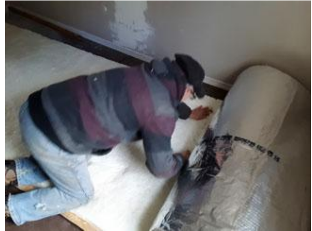
John Boy Delaney cuts the insulation to be installed in our next Fuller Center home, number 23, which is located in Smelterville.
