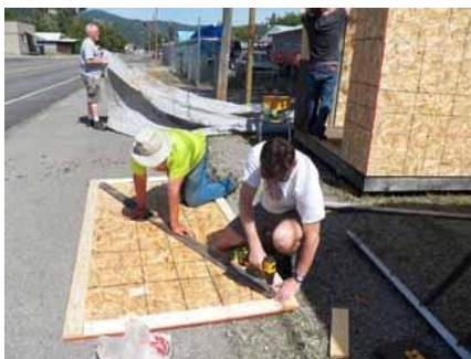
While one crew worked building a shed, others finished painting outside on the front of the store and another group painted the floor inside.
