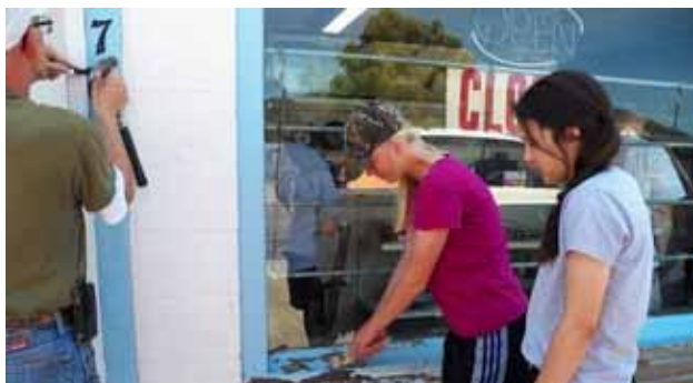
John Delaney removes the store numbers as some kids scrape the peeling paint from around the windows.
