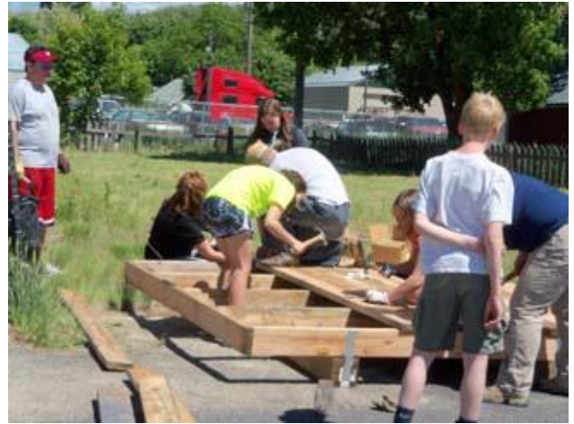
Holy Family Catholic School youth learn how to pound nails while building the floors for sheds.
