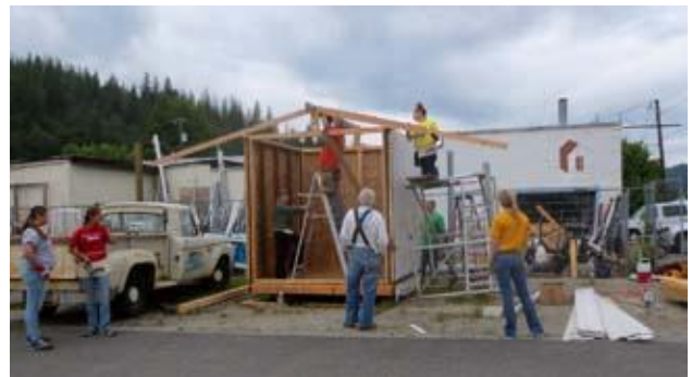
Idaho Servant Adventurers from Minnesota, who stayed up the river at the Shoshone Mountain Retreat, spent four days working on projects around our community. This group is learning some carpentry skills while building a shed that we can sell at the ReUse Store.
