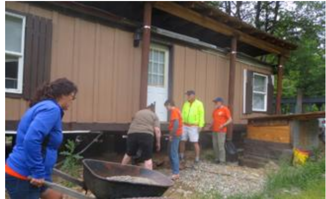
A crew of 6 Fuller Center for Housing Bike Adventurers work with Krista Kirby moving gravel, donated by Zanetti Brothers, around the posts that hold up the snow roof over her replacement trailer home.
