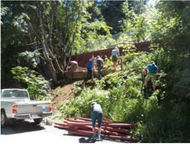
Jim Taylor of Taylor Made Construction shows volunteers from the Holy Family Catholic School group how to dismantle the damaged retaining wall.
