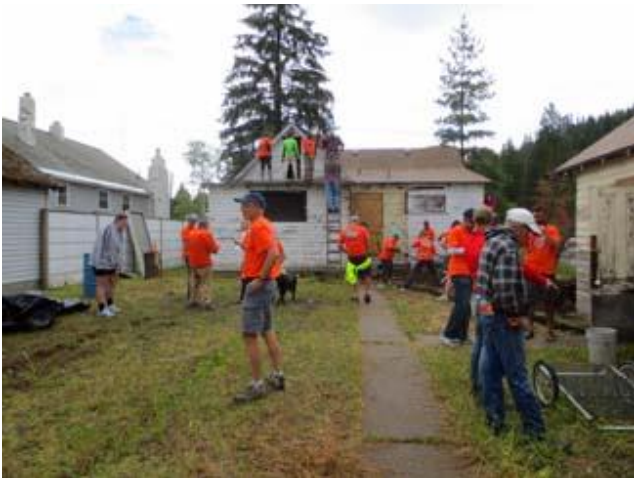
They start finding projects to work on at John "Boy's" future home in Osburn. One of the first things will be tearing off the flat roof and walls of the room on this side where some are standing. This was where the whole ceiling was falling in and the floor was warped.
