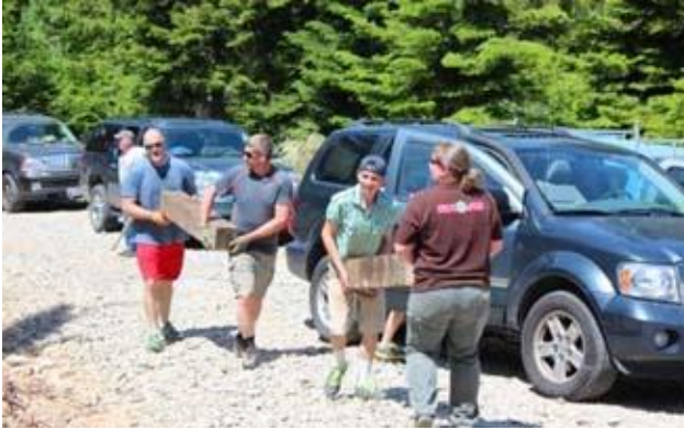
Volunteers move the railroad ties in place to make a terraced hillside in front of the home.
