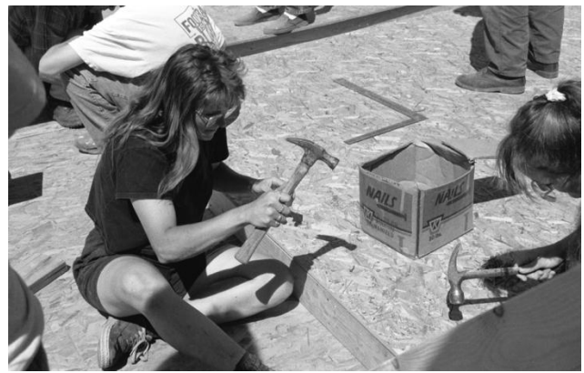
Anne Duncan and Sally Davis develop nailing skills while building the Duncan's walls. Photo by William Bunton
