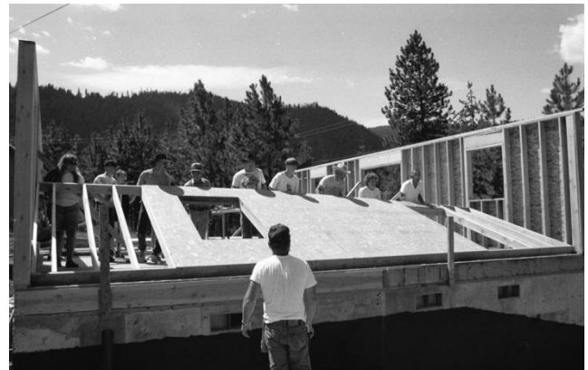
UP IT GOES! While Sally Davis watches from behind, Jim Campbell checks the wall's alignment as Mary Davis, Mike Spencer, Drago Duncan, Wayne McPeak, Casey Duncan, Dan Davis, Verne Blalack, Chris Campbell, and Ron Booth raise a wall on the Duncan home.
