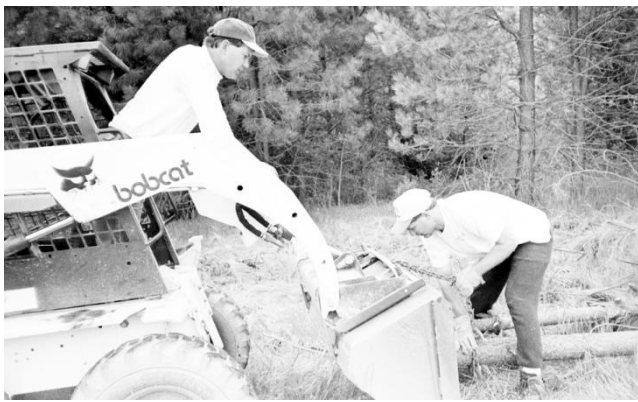
Randy Seaton and Terry Seaton clear the logs from the Duncan home site after Dick McPeak, Construction Supervisor, felled the trees. Photo courtesy of Shoshone News-Press and Bunton Studios
