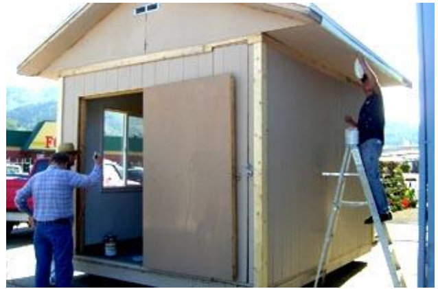
Last May, Verne & Bob discuss the construction of the “Little Shop’ while Skyler Wilburn paints the soffits. We still need to sell about 70 tickets before we can raffle it. In addition to the other businesses who are selling tickets, Kellogg Lumber Co, Ace Hardware, and Building Maintenance now have them for sale. Remember, there is an offer of $1000 for the winning ticket if you don't want the building. Tickets are $10 ea. or 6 for $50
