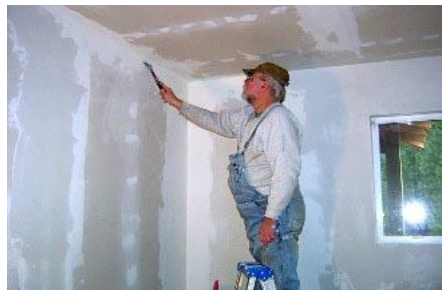
Swede Little smoothes the mudded walls in preparation for painting at the Lake site.
