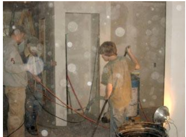
Ian Hauser, at right, helps his cousin Chris Leetch and Bob Larson with the insulation. Ian helped break up the bags of insulation before it was fed into the hopper to be blown in the attic. The spots in the photo are from the insulation floating around
