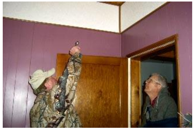
Electrical inspector, Doug Morfitt, checks out the wiring in the Pelham house in Mullan with Verne. Boxes for the ceiling lights and most of the outlets needed to be replaced.
