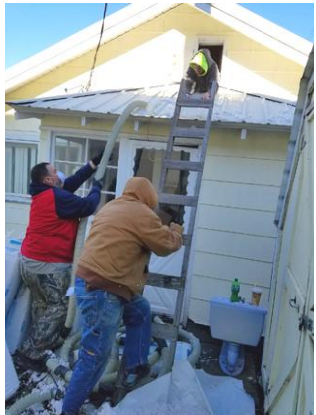
After the hose accidentally got away from John Boy, slid off the roof and sprayed a shower of insulation around outside, Mike and Verne get the hose back up to him.
