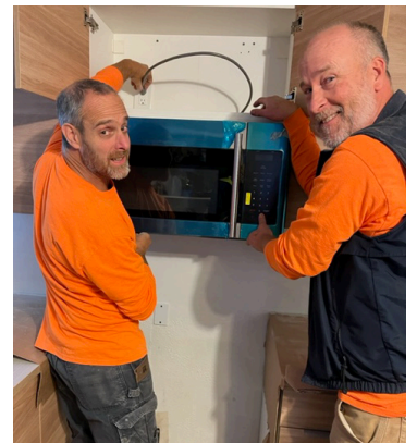
The microwave is installed as part of the kitchen remodel last month
