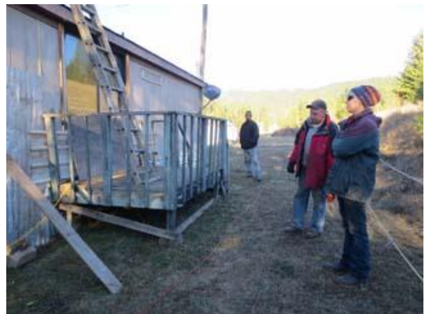
CJ, Rick & Debbie discuss the removal of the back porch. The immediate concern is freezing pipes; the porch can be rebuilt next spring.
