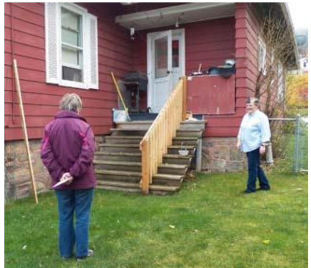
Ellie Arguimbau admires Mary Kay Hanson's new porch railing installed by Kevin Hutchings.
