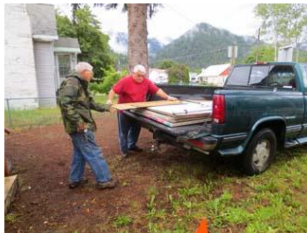
Verne helps Steve Milot unload the building materials he donated. Verne & John "Boy" moved it into the Osburn house where it will be used in the renovation process.
