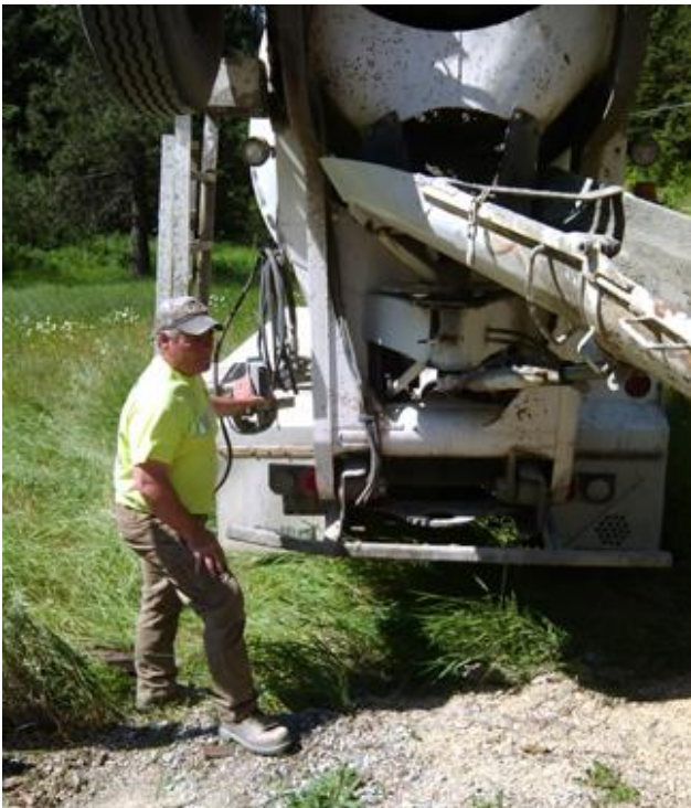
Our crew was very impressed with Zanetti's concrete truck driver, Ken Deaton, who could place the spout within a half inch. Although there were wheelbarrows handy, none were needed, and the pour took much less time than expected.
