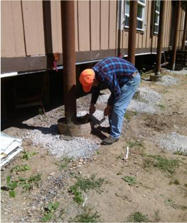
Verne Blalack trowels the top of the concrete poured around the support posts of the snow roof erected and donated by David Rust over Krista Kirby's trailer home.
