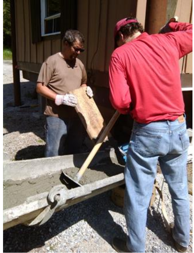
When home for a family reunion, the Blalack brothers, George and Tallis, work the concrete down the chute into the holes around the posts. They grew up helping their father, Verne, install chain link fencing throughout the valley.
