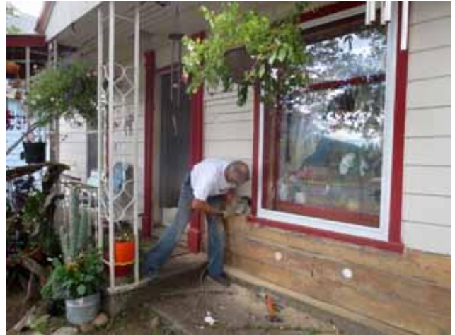
John Delaney sands the old peeling paint off the Souza home while Verne begins priming the opposite gable end.
