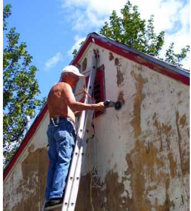
With his ladder secured to the eave, Verne uses a heavy sanding disc to remove the mostly peeling lead paint from the Sousa home.
