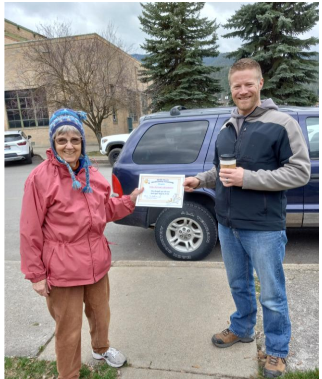
Bob Whitman captures this shot of Ellie Arguimbau presenting a certificate to Clint Kunze when the Greater Blessings committee met with him to evaluate a leaking roof. Clint is the coordinator of the Idaho Servant Adventurers who come in different groups for several weeks each summer to help in the valley. We are delighted to work with them on our projects.
