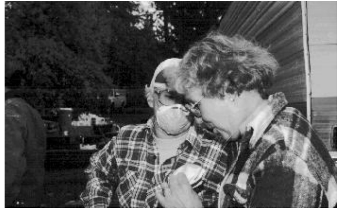
Nancy Hardy and Gladys Trecker don their masks before installing insulation during "Make a Difference Day"
