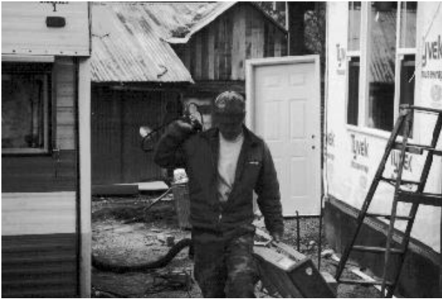
Electrician, Dan Reardon, walks past the windows sold to us at an incredible discount and installed free by Shoshone Glass and doors donated by Kellogg Lumber Co.
