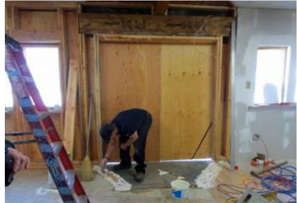
Kevin Hutchings uses Fix-All to level the floor in front of the new door space.
