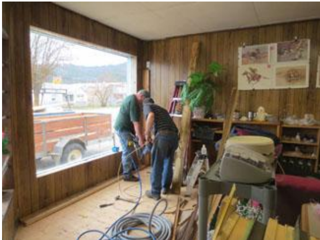
Jim Taylor and Kevin Hutchings begin the process of removing wall board so as to be able to replace the single pane front window.
