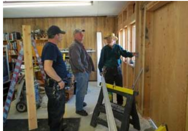
Kevin & Verne explain to George Hemphill of Electric & Supply their vision of the remodeled front wall. George and his crew will install the wiring. Photos by Judy
