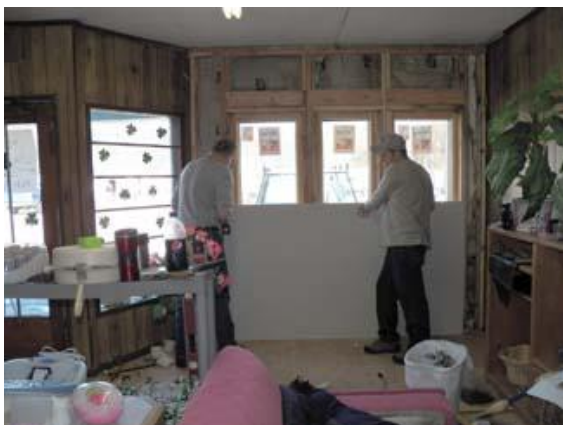
Chris Leetch assists Joe Wolford as Joe installs new insulation and wall board around the new windows.
