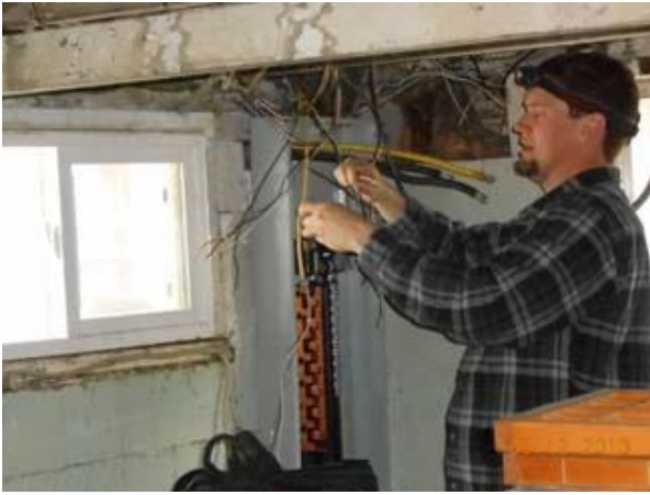
Josh Haralson installs a new breaker box and connects all the loose wires to it at the Burbridge Greater Blessings job.
