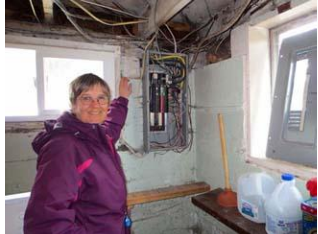
Greater Blessings Committee member, Ellie Arguimbau, points to the rat's nest of wires going to the fuse box at Diana Burbridge's home.
