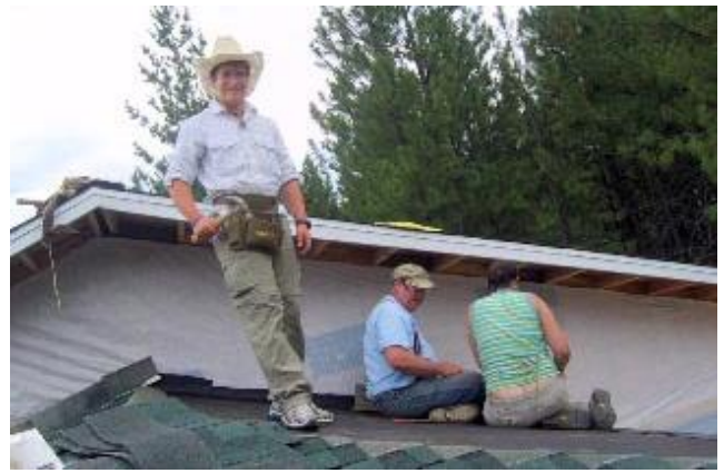
Jim Taylor, of Taylor Made, (center) teaches the Shoshone Base Camp Youth how to install roofing and siding.
