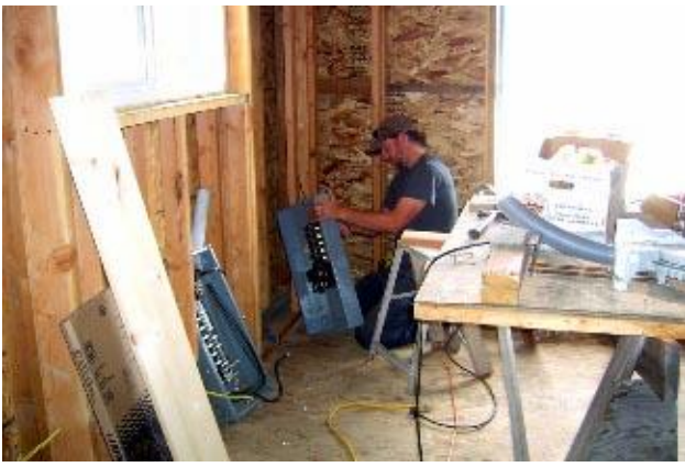
Gary Pruiksmas from Crown Electric installs the circuit panel at the Lake home.
