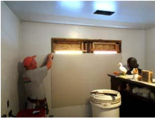
Rick Gilbert teaches Hudson Bartlett how to install wall board around the kitchen windows at the Osburn house. He stressed the need not to pound too hard but to make the nails flush and smooth with the wall.
