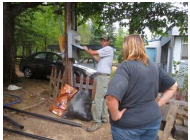
Electrician, Josh Haralson for Amp Electronics, tells Krista that the power pole will have to be replaced and set on the other side of the trailer since the snow roof will be 6 feet higher.
