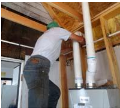
John "Boy" Delaney installs insulation behind the pipes of the inline water heater in the Osburn house. Sheetrocking behind it was tricky.
