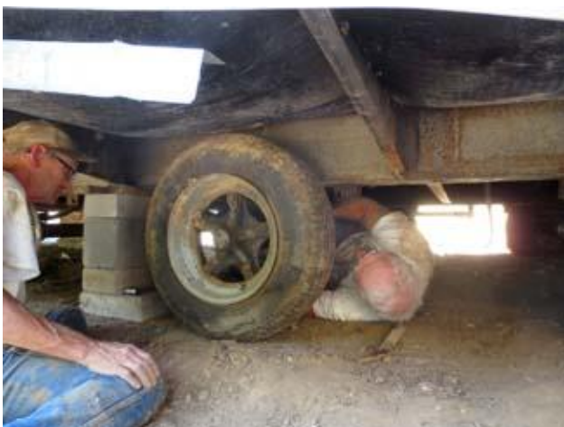
John "boy" and Verne remove one of the axles from under the trailer so Krista could get to the piping above the axle. They were both very dirty and tired that night. Ron Ireland removed the other two.
