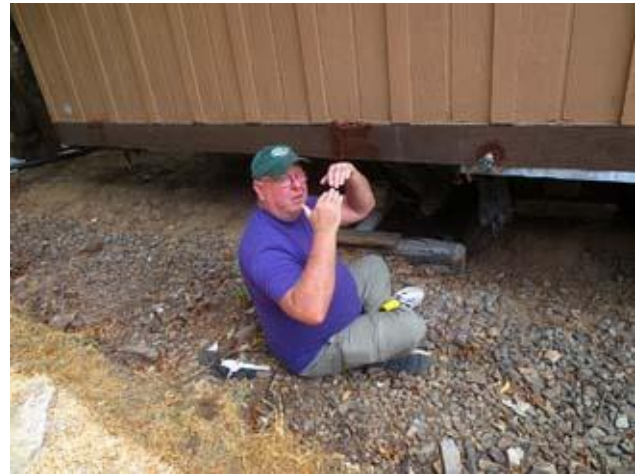
Jim Taylor of Taylor made Construction stops by to tell Krista how to install the plumbing herself. We appreciate the help and advice given at Building Maintenance in determining what fittings Krista needed.
