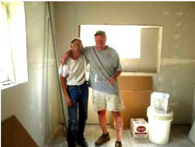
Another day, Rick teaches John "Boy" how to do the mudding before taping. John "Boy" spent that night filling in all the nail holes and seams throughout the house to be ready for taping the next day.
