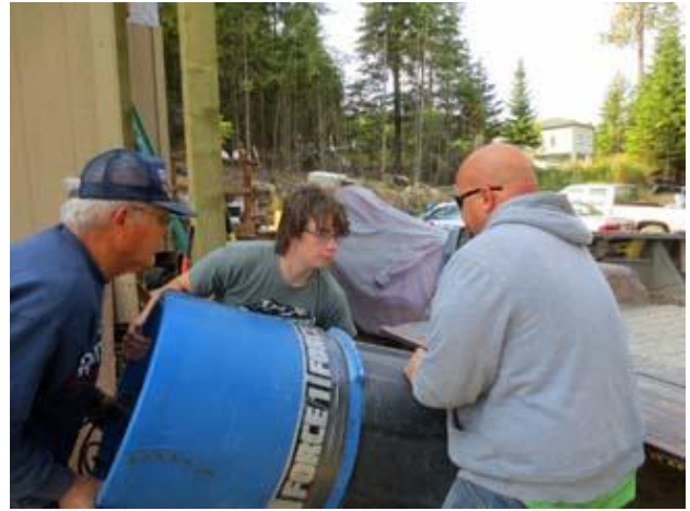
Verne, Nate Galford, and Joshua Mace load the insulation hopper after installing insulation under the house. Work continues at the Mace home on drainage around the house and skirting installation.
