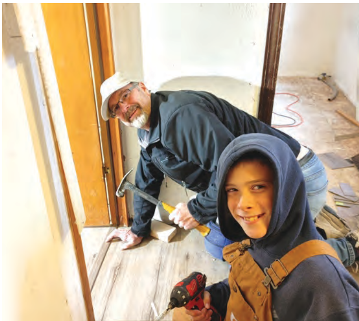
Ken Morris and Jedidiah Braunstein installed the new vinyl-plank flooring in the trailer.
