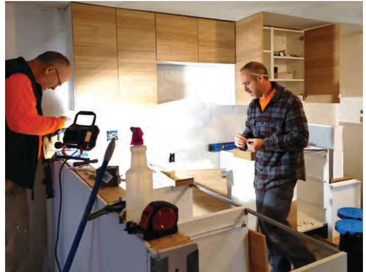
Bryan Weed and Joshua Braunstein work to install the kitchen cabinets that their group donated to Brian's trailer.
