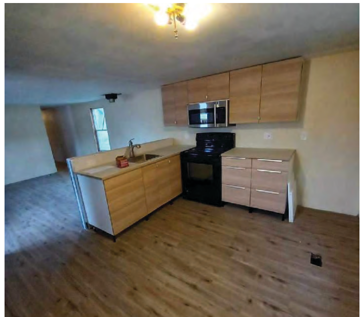
The remodeled kitchen with new cabinets, sink and faucet, range and microwave.
