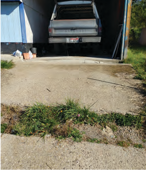
Michael's driveway which has shifted, causing a significant gap in the concrete.
