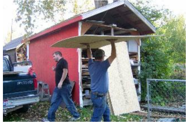
Josh Baugh and Kevin Hutchings unload T-111 siding donated by The GUESTHOUSE Inn & Suites.
