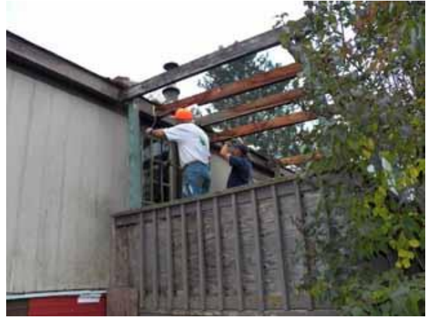
Verne & Rick Wood remove the roof from the front porch of Debbie Bornitz's home before her main roof could be replaced. Photo by Judy
