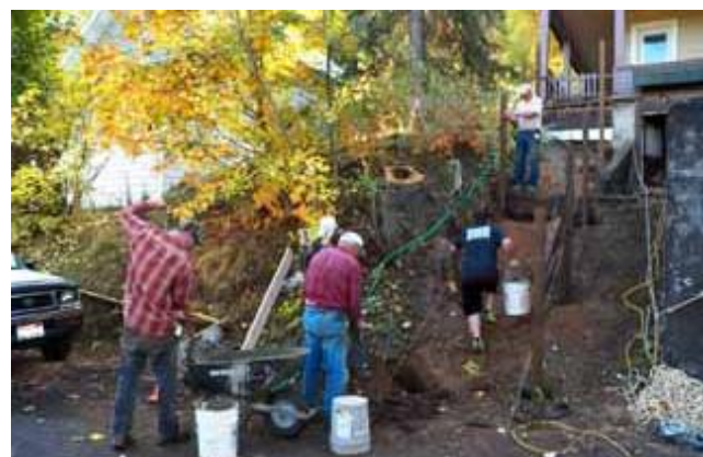
Jared Kitchen packs a bucket of concrete up the hill from the mixing crew of CJ Leetch & John Delaney to Rick Gilbert where it is poured around a post. Verne is digging a new post hole. Photo by Judy
