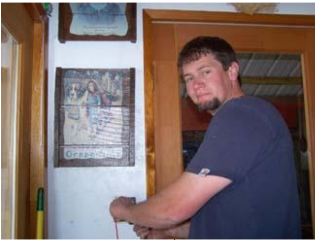
Josh Haralson finishes the 2 nd phase of wiring for the Burbridge Greater Blessings Project. Photo by Lanora Helbig
