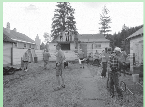
2016 Adventurer's start finding projects to work on at John "Boy's" future home in Osburn. One of the first things will be tearing off the flat roof and walls of the room on this side where some are standing. This was where the whole ceiling was falling in and the floor was warped.
