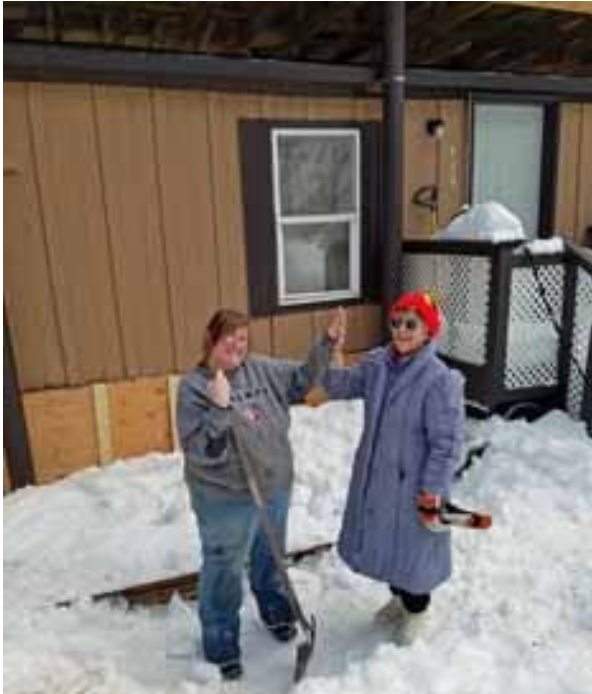
Krista Kirby and Judy Blalack do a high 5 after finally getting the skirting installed around the trailer. With just a few things left for her to finish, we will be able to get insurance on the property and have a final inspection. Then we can have a dedication after the snow melts so there will be parking.
