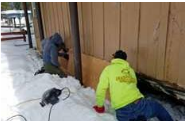
In addition to screwing the skirting in place, Krista & John cut the vent holes. Photos by Judy
