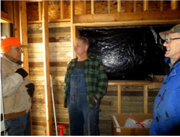
Verne & John “Boy” meet with Jeff Crawford of Systems Design about installing a furnace in the Osburn house.
