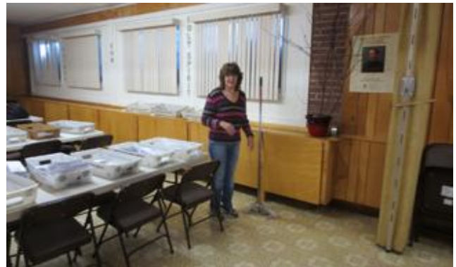
Linda Amonson mops where water seeps up through the floor in St. Rita's Parish Hall where we do the mailing. Note in the top photo how much snow has slid off the roof next to the window.
