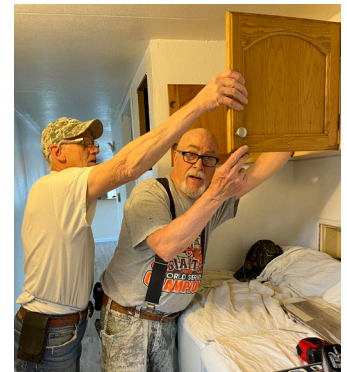
John Boy and Glen Smith install a cabinet above the washer and dryer in Brian's trailer
