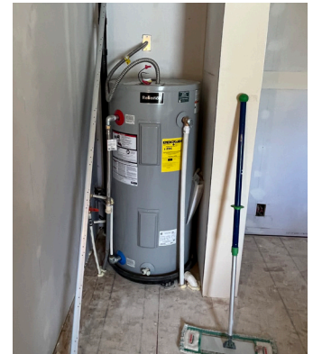
The new water heater installed in Brian's trailer
