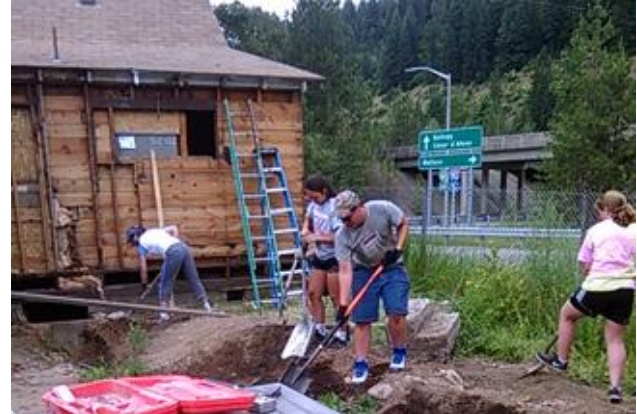
Members of one of the Servant Adventurers from Shoshone Mountain Retreat work on the Osburn house. Here they are covering the electrical conduit laid in a ditch from the house to the garage.
