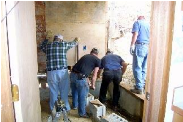
Bernie Ussery, Kevin Hutchings, Lew Young and Milo Johnson work to level a wall at the Pelham home.
