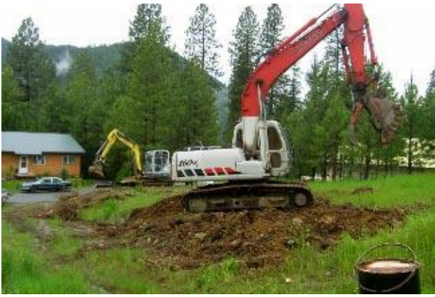
Keith Sims, of KASCO of Idaho, sent Stan Darliss & T. J. Trecker with track hoes to excavate the foundation for the Kriedeman home at Sunny Slopes. Photos by Judy
