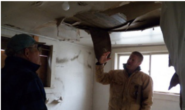
Verne Blalack and Clint Kunze (Servant Adventurers Coordinator) in the back room with the ceiling falling in and black mold
