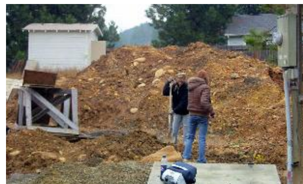
Helpers, Carissa Gohl and Penny Welsh, shovel fill into a trench to cover the pipes at the Kriedeman site.
