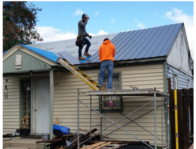
Son, Bill Prince, and son-in-law, Chris Sears, finish the roof on Luke and Caroline Prince's home. Only roof cap left to do.
