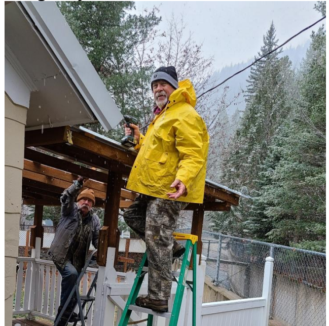
Chuck Carlson helps Glendon Smith work quickly to finish Dawn's porch while the weather holds.
