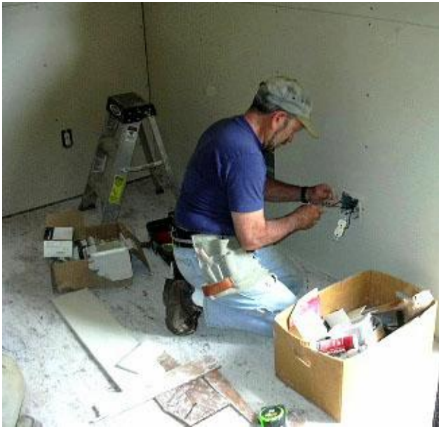
RV'er, Marv Edelstein works on an electrical outlet. Photo by Diane Gravlee
