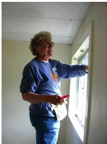
Audrey Ussery works on a window in the Pelham home. Photo by Diane Gravlee
