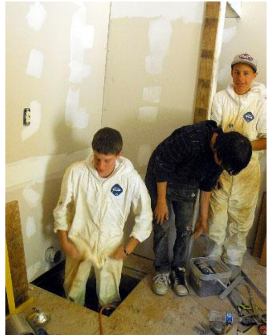
Shoshone Base Camp Servants brush off dust after working under the floor.
