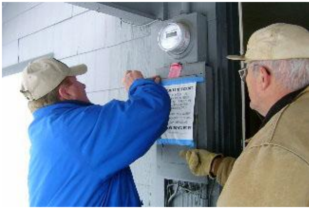
Verne watches as Electrical Inspector, Doug Morfitt, checks the electrical box and wiring at the HUD home in Smeltonville. If a building has been vacant for a year, the inspector must approve having AVISTA turn on the juice.
