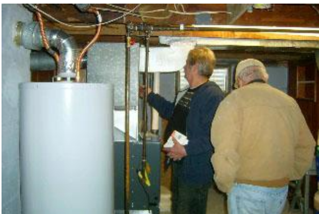
Jeff Crawford finishes installing a new furnace & water tank in the Kriedeman home site. Verne notes it is great to have heat and water during the rehab!
